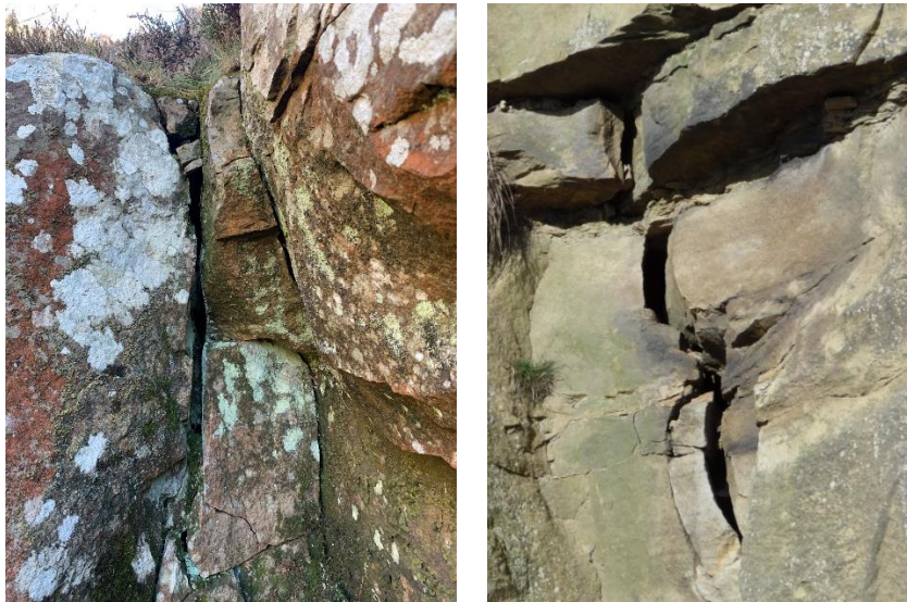
Figure 3a-b Fissures noted within quarry face
